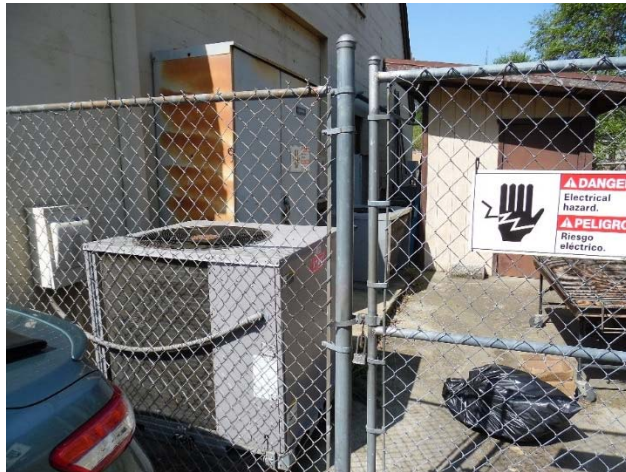
Figure 16 - Town Hall HVAC Units
