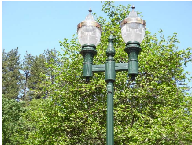
Figure 160 - Parking Lot Lighting.
