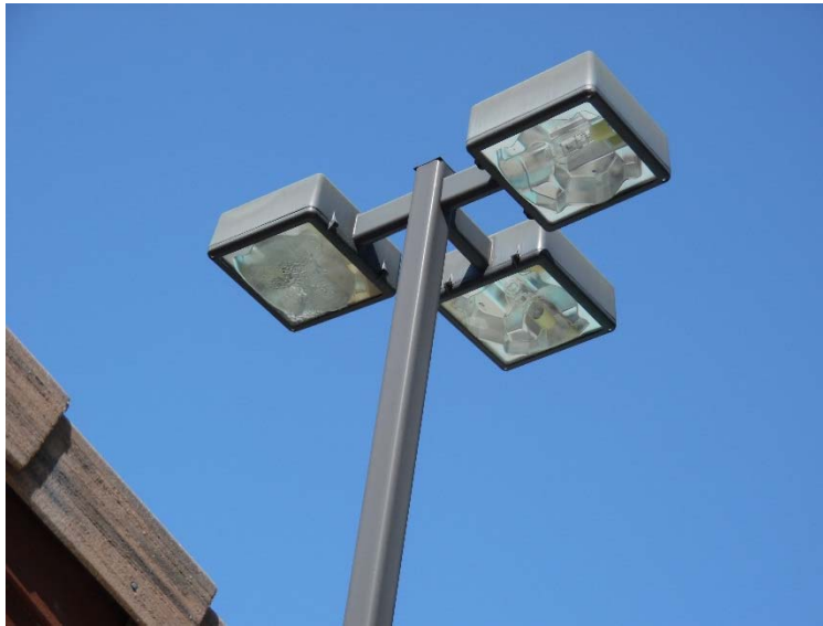
Figure 194 - Pool Deck Lighting.
