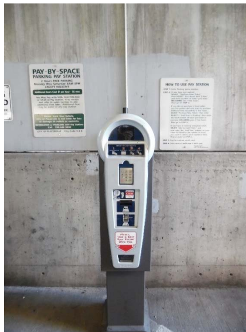
Figure 8 - Parking Metering and payment Station
