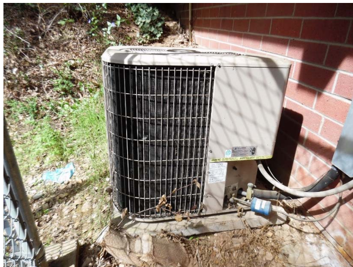
Figure 12 - Police Department HVAC Unit
