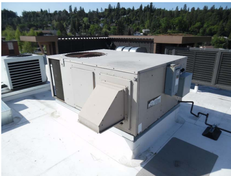
Figure 6 - City Hall HVAC Unit
